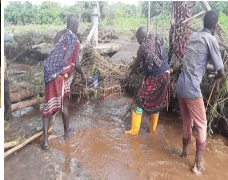
Some of the Mtipule community members clearing the area around the well after a heavy rain destroyed the well.
